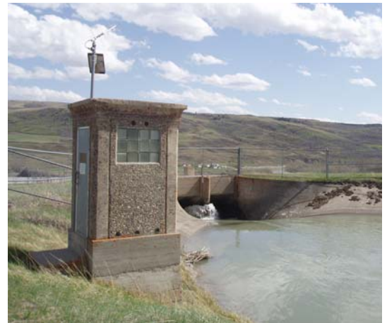
Gauging station upstream of the siphon that delivers water to the Milk River from the St. Mary River. Photo: S. Riemersma
