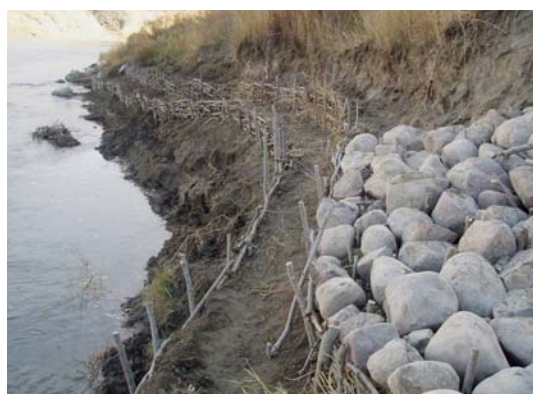
Bioengineering project on the Oldman River. "Live stakes" are planted while dormant.
